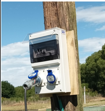
One of the new improved power boxes
